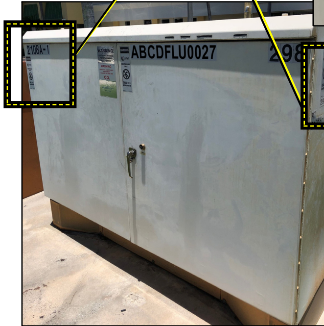
FUJITSU 6200 CABINET (OUTSIDE VIEW)
