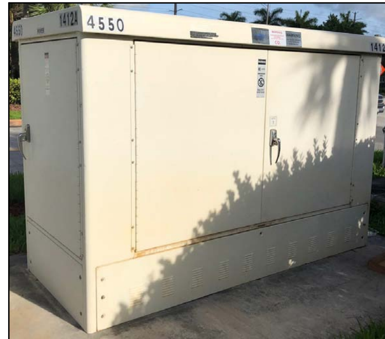
LSC-2030 CABINET (OUTSIDE VIEW)
