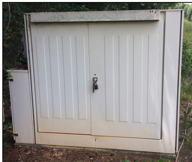
NORTEL OPAC / OPM CABINET (OUTSIDE VIEW)
