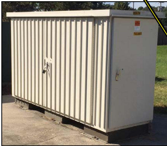
LS2000 CABINET (OUTSIDE VIEW)
