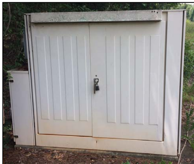
NORTEL OPAC / OPM CABINET (OUTSIDE VIEW)
