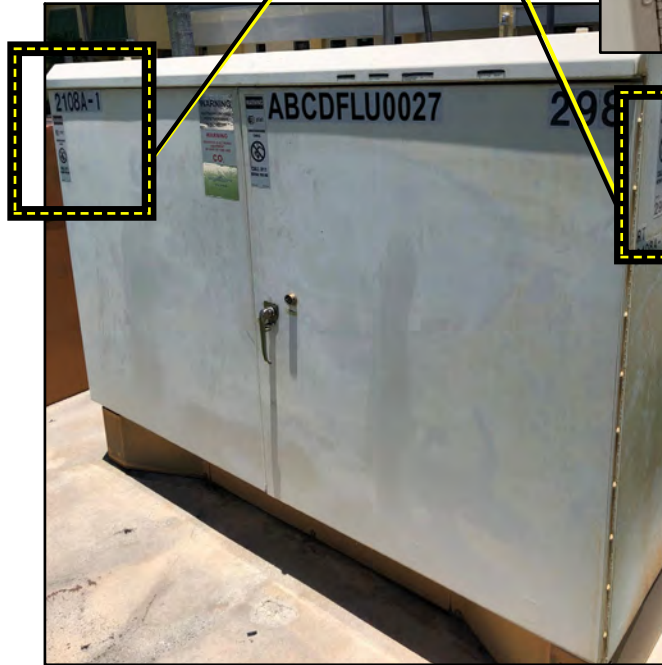
FUJITSU 6200 CABINET (OUTSIDE VIEW)
