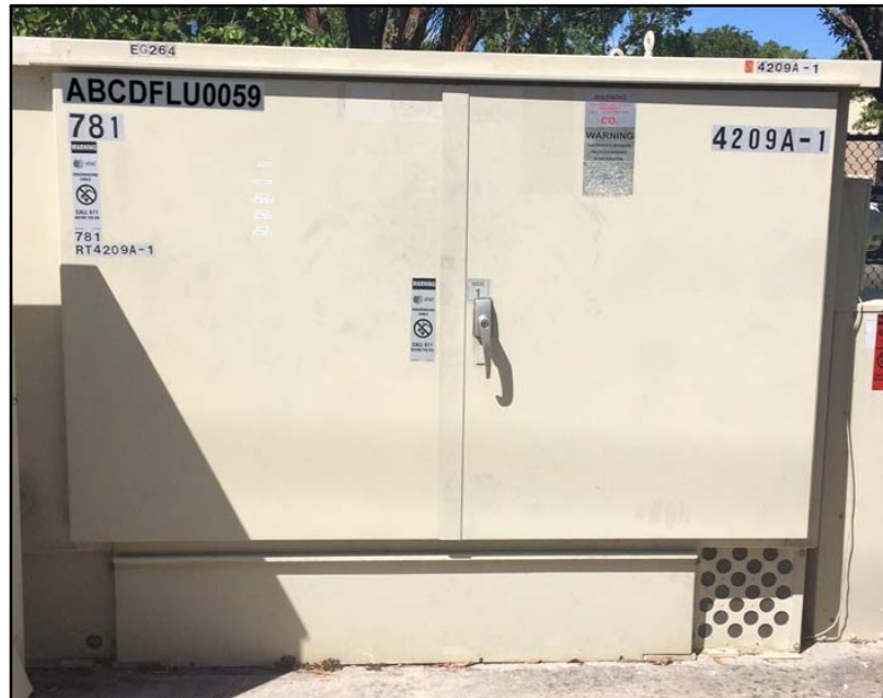
LSC-2020 CABINET (OUTSIDE VIEW)
