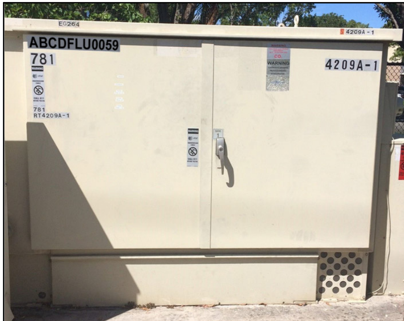
LSC-2020 CABINET (OUTSIDE VIEW)
