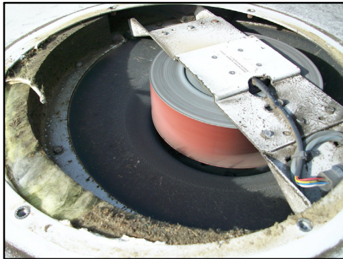
SOLAR SHIELD ON CABINET (TOP FAN)
