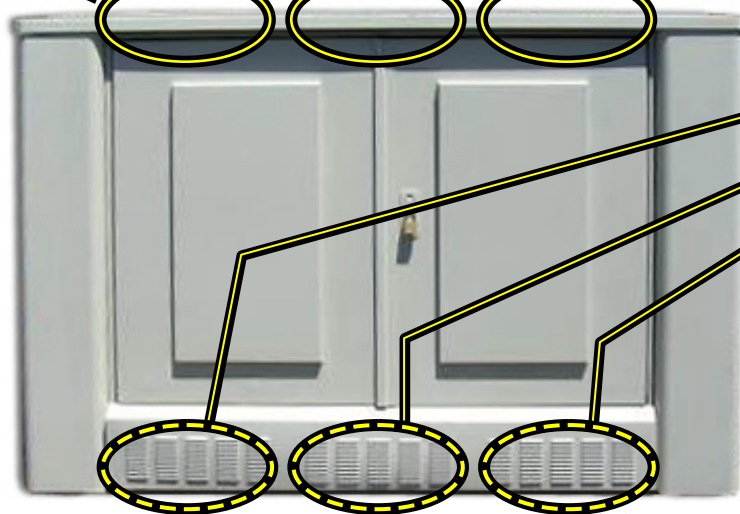
MESA 6 CABINET (OUTSIDE VIEW)
