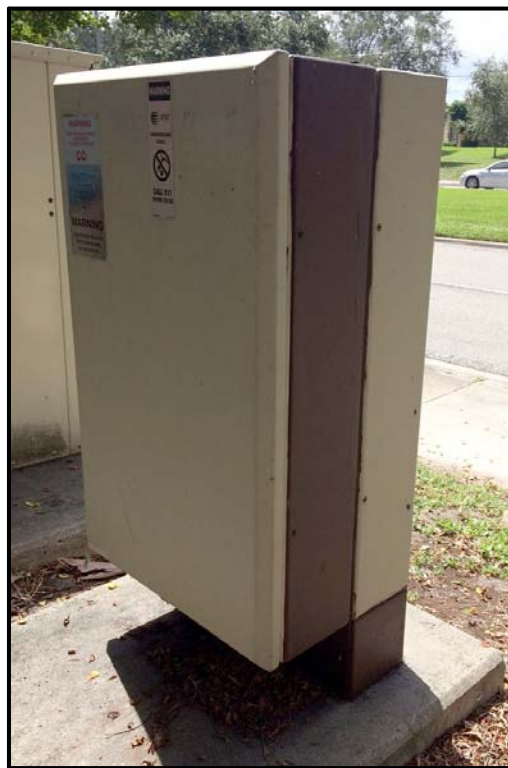
36B CABINET (OUTSIDE VIEW)
