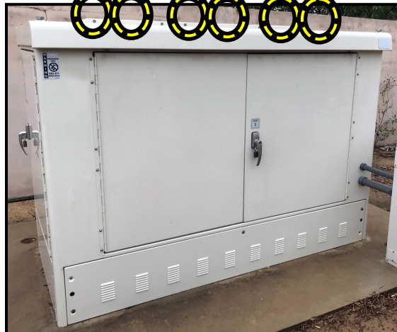
LS2016 CABINET (OUTSIDE VIEW)
