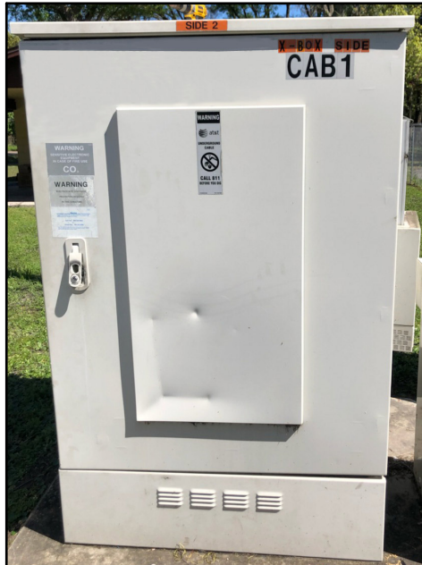
MESA 384 CABINET (OUTSIDE - FRONT VIEW)
