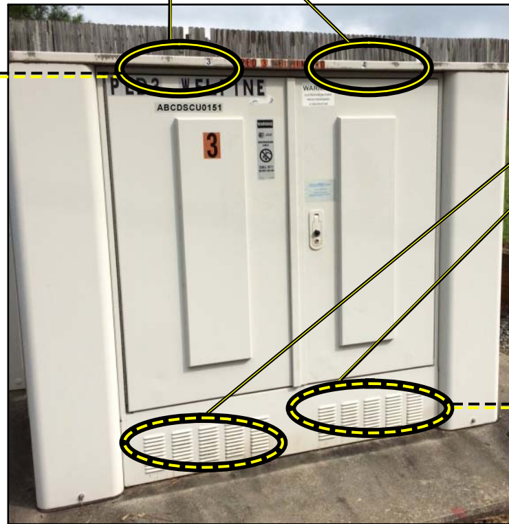
MESA 4 CABINET (OUTSIDE VIEW)
