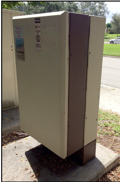
36B CABINET (OUTSIDE VIEW)
