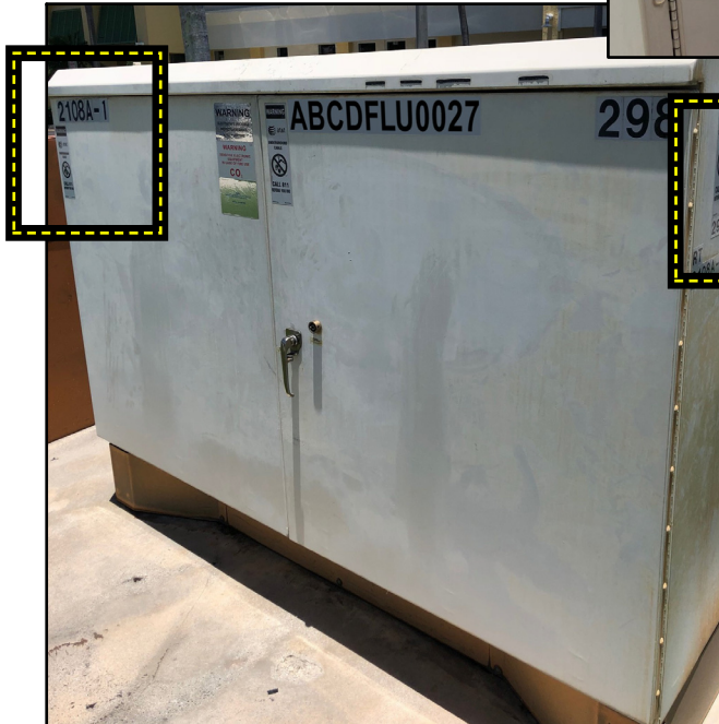
FUJITSU 6200 CABINET (OUTSIDE VIEW)
