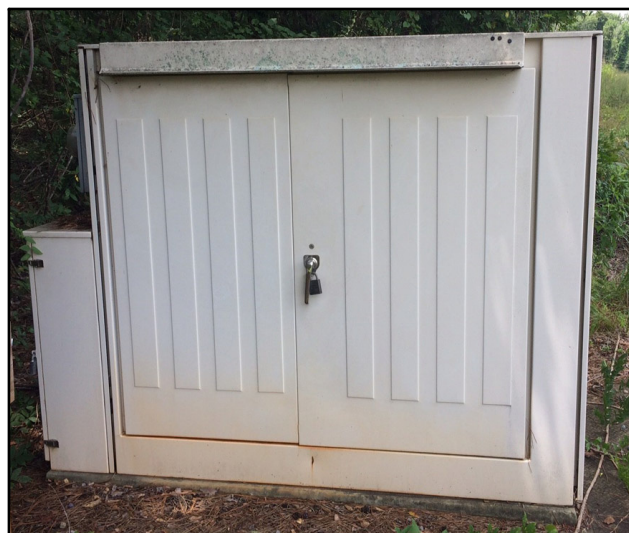
NORTEL OPAC / OPM CABINET (OUTSIDE VIEW)
