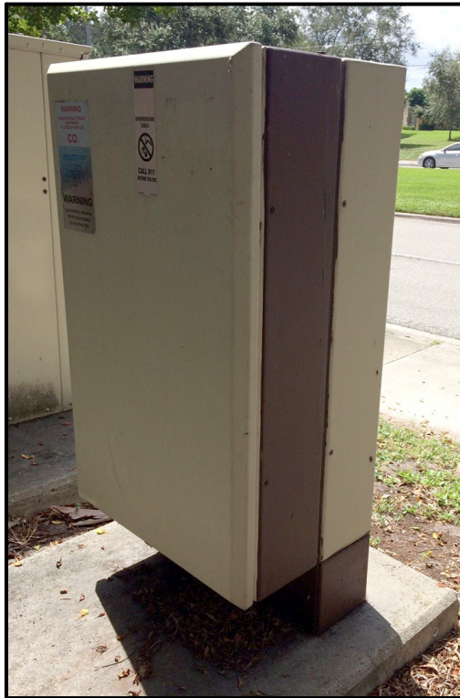
36B CABINET (OUTSIDE VIEW)
