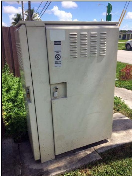
COMMSCOPE 52B CABINET (OUTSIDE VIEW)
