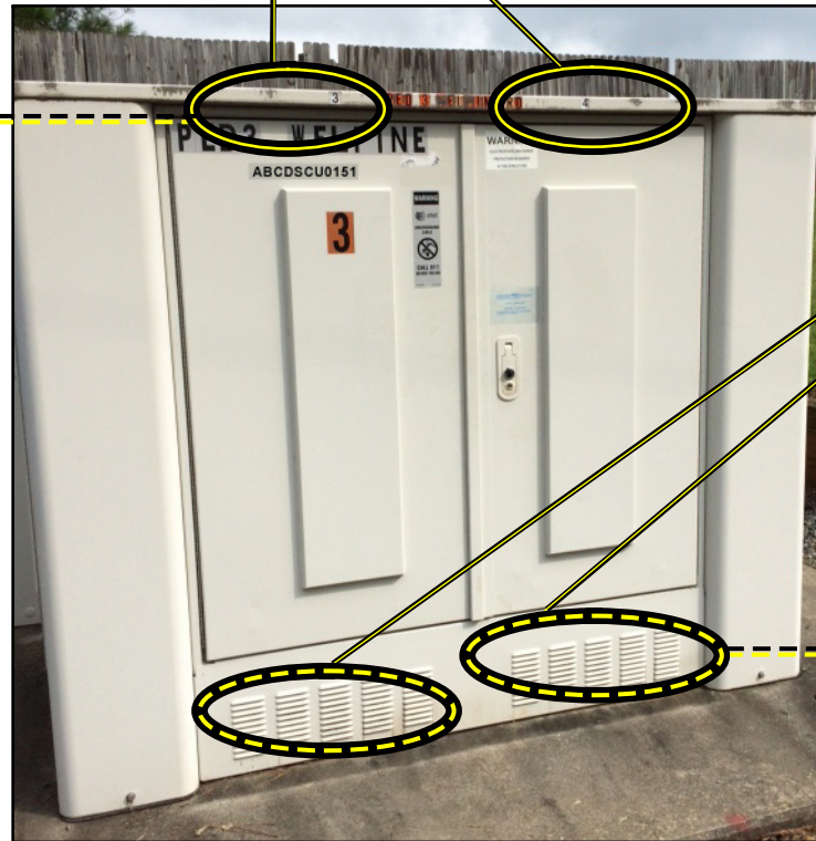
MESA 4 CABINET (OUTSIDE VIEW)
