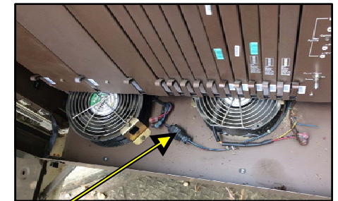
TRAY VIEW - FANS w/ WEATHERPROOF PLUG (2) FANS PER TRAY
