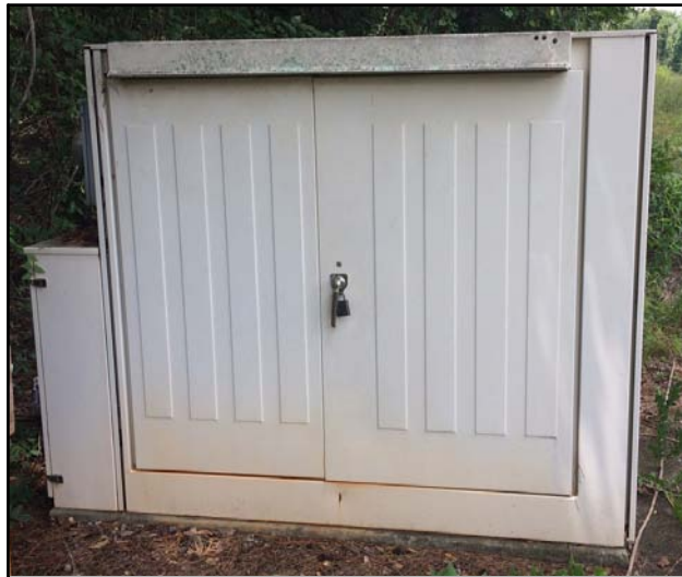
NORTELOPAC / OPM CABINET (OUTSIDE VIEW)
