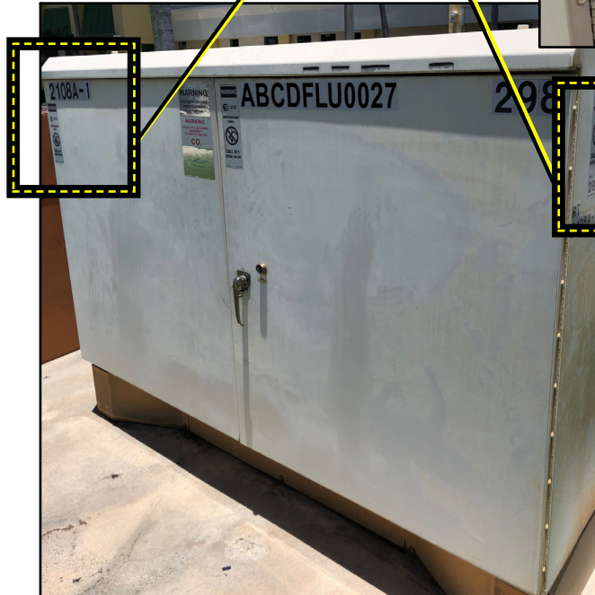
FUJITSU 6200 CABINET (OUTSIDE VIEW)
