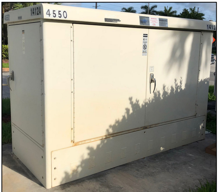
LSC-2030 CABINET (OUTSIDE VIEW)
