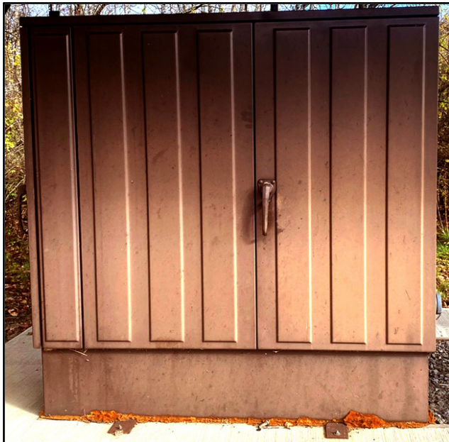
NORTEL DMS OPM CABINET (OUTSIDE VIEW)
