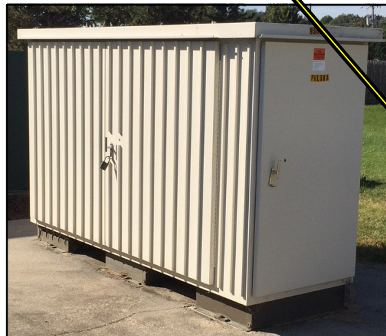
LS2000 CABINET (OUTSIDE VIEW)
