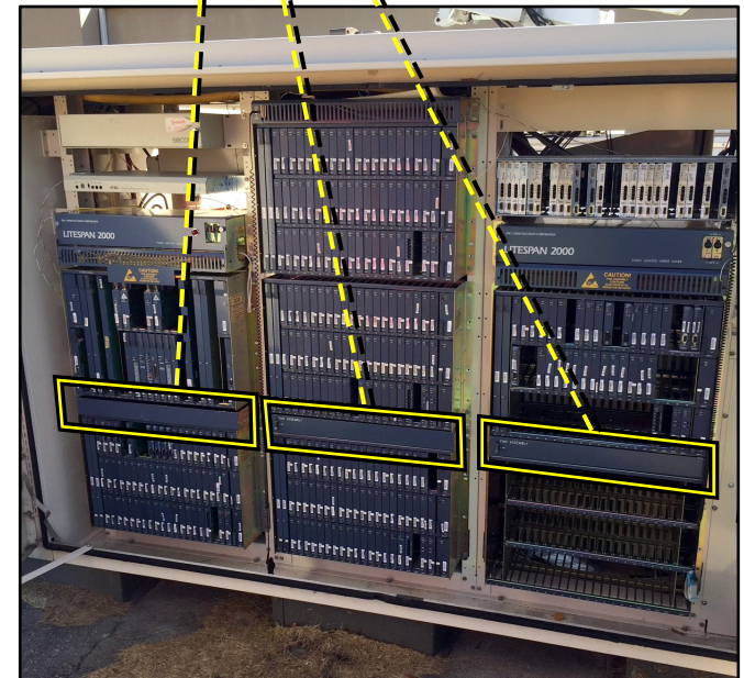
LS2000 CABINET (INSIDE - FRONT VIEW)
