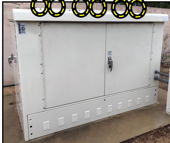
LS2016 CABINET (OUTSIDE VIEW)
