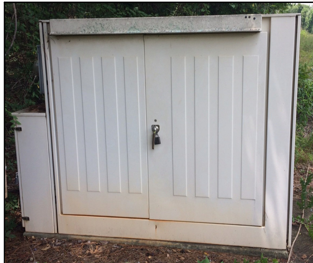
NORTEL OPAC / OPM CABINET (OUTSIDE VIEW)
