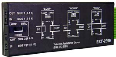
EXT-239E T1 Line Repeater Access Board w/ Bantam Jacks 12 STATE SOUTHEAST ATT.100001303 ATT.100001303
