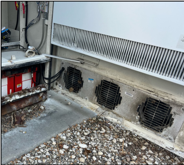
COMMSCOPE ALP 448/248 CABINET
