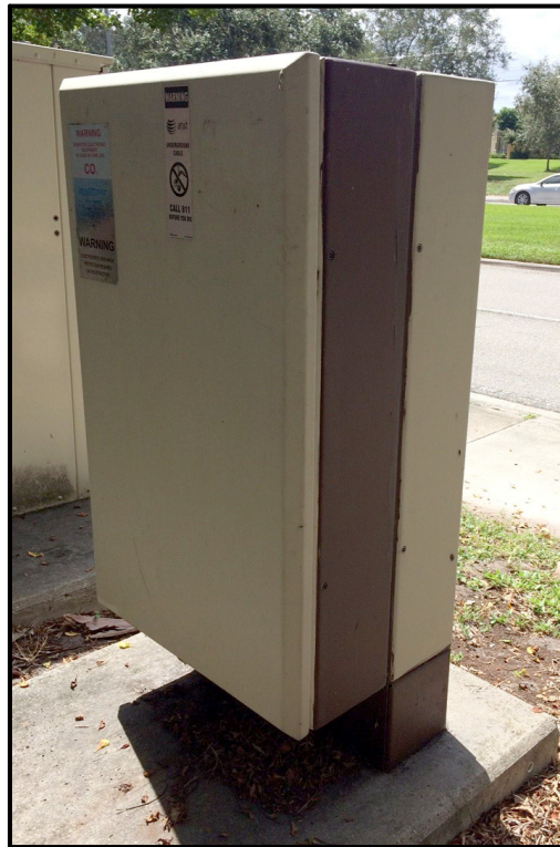
36B CABINET (OUTSIDE VIEW)
