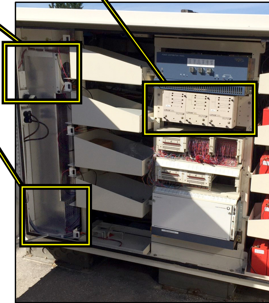
LS2000 CABINET (INSIDE - BACK VIEW)
