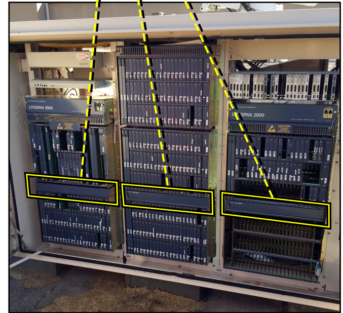
LS2000 CABINET (INSIDE - FRONT VIEW)
