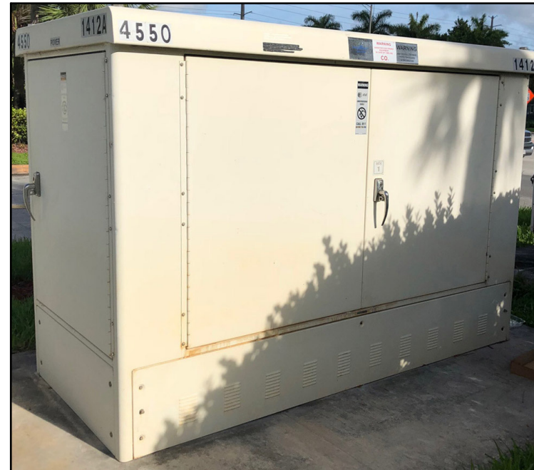
LSC-2030 CABINET (OUTSIDE VIEW)
