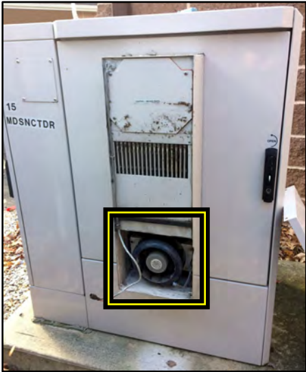
VIEW OF A009 CABINET w/ FAN COVER PLATE REMOVED
