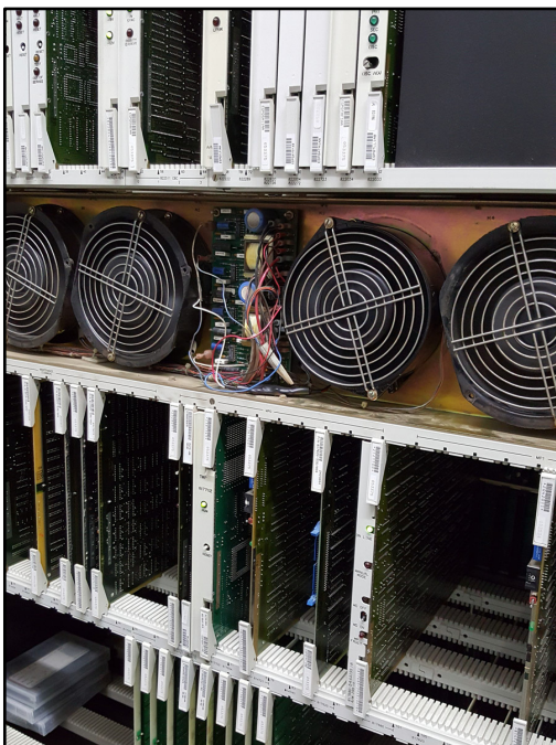
STROMBERG CARLSON DCO CMF / DTF BAYS (w/ 4 EXISTING FANS)
