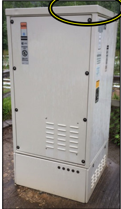
MESA 768 CABINET (FRONT VIEW)
