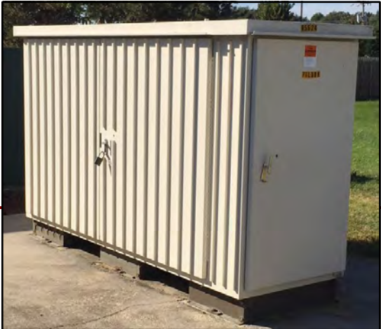
LS2000 CABINET (OUTSIDE VIEW)
