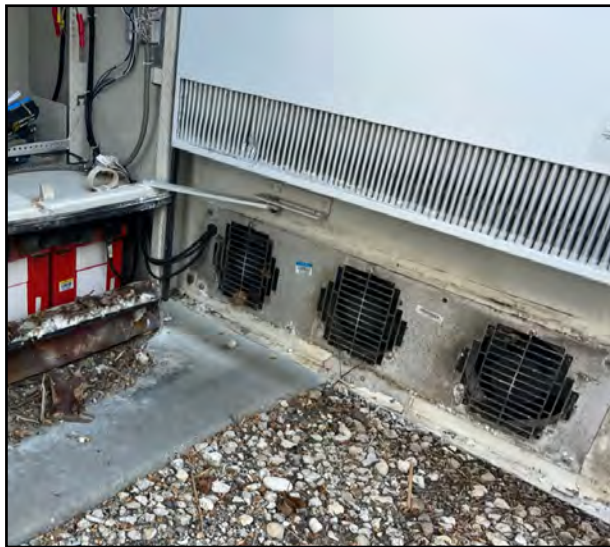
COMMSCOPE ALP 448/248 CABINET
