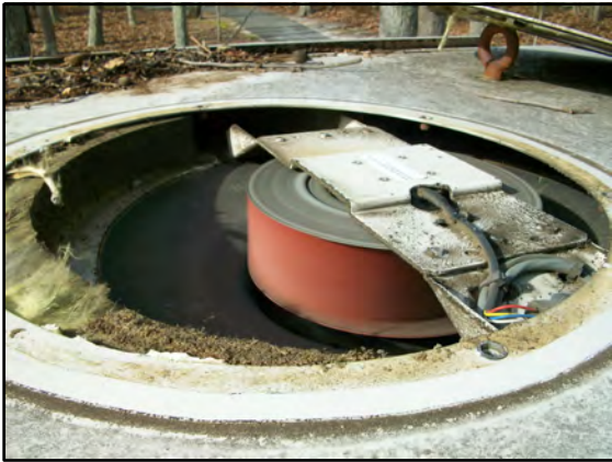
TOP / ROOF (SOLAR SHIELD) OF MESA CABINET w/ EXISTING HEAT EXCHANGER
