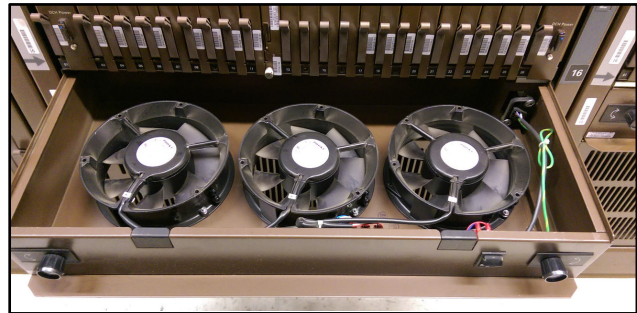
DMS-100 NTRX91AA FAN UNIT w/ EXISTING FANS
