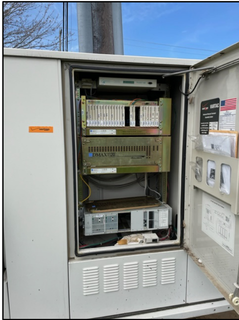
MESA BRIDGE CABINET (FRONT VIEW)
