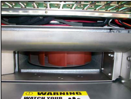
INSIDE / BOTTOM VIEW OF MESA CABINET w/ EXISTING HEAT EXCHANGER
